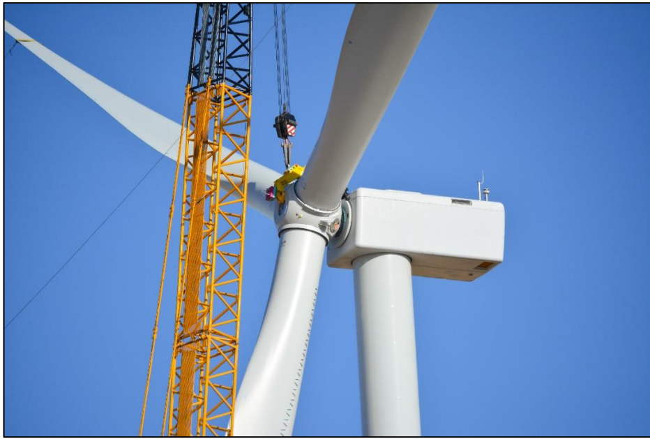
Figure 3. Installing the Rotor on CCPPD's Wind Turbine. Courtesy of Bluestem Energy Solutions.
