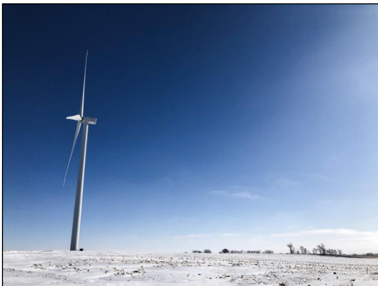
Figure 2. CCPPD's Wind Turbine. Courtesy of Bluestem Energy Solutions.
